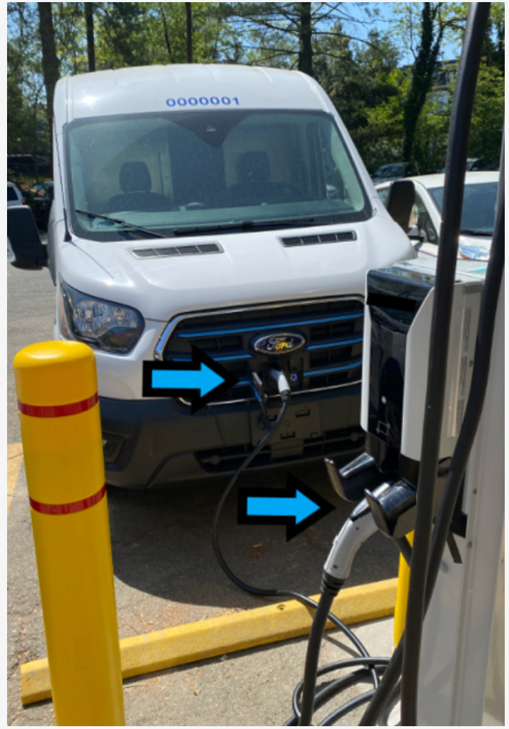
Figure 2. Examples of Electric Vehicle Charging Station Heads
